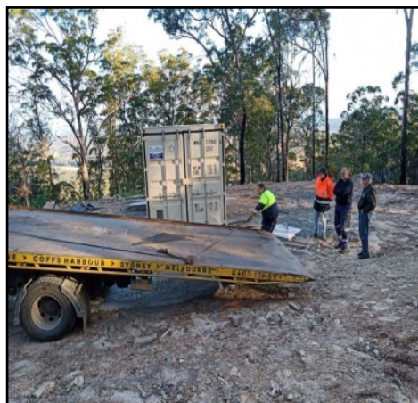
Rob VK2CRF, Lyle VK2SMI and Arthur VK2ATM oversee the positioning of the equipment shed.
