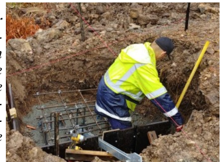
Mast Anchor block form-work South West guy. Note the large size of the form-work compared with the contractor.
