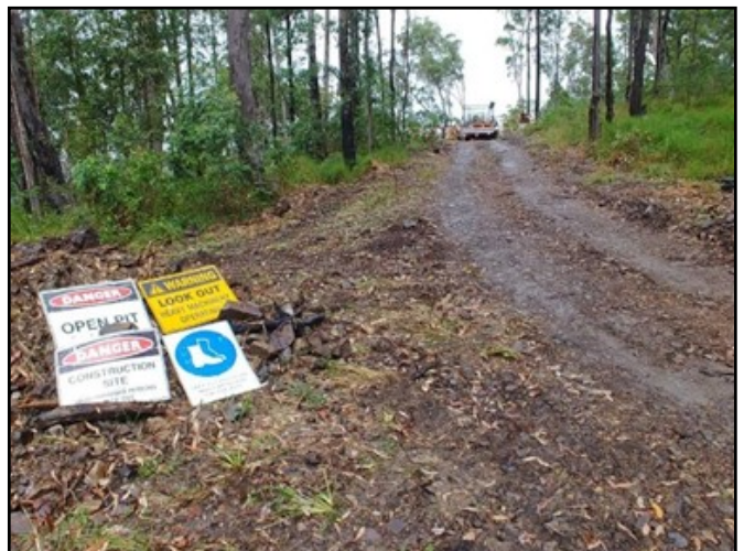
A road entrance is established ready for the next phase of construction.
