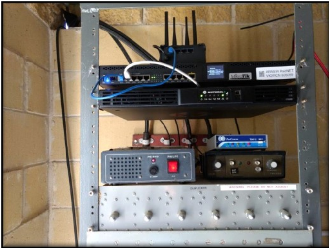
Repeater installed in rack
