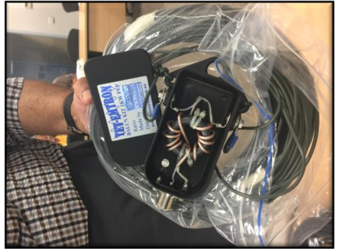
Labels and balun assembled
